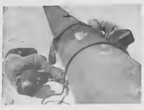
Members of a Tappin welding crew weld two sections of the pipeline on the desert near Qaisumah. The final main line weld was completed in September 1950. Arab workmen learned new skills readily.
